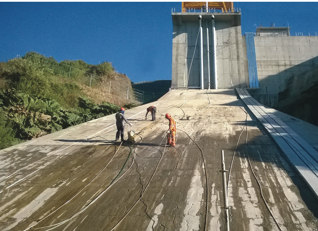
Rucatayo Hydroelectric Power Plant, Puyehue, Chile
